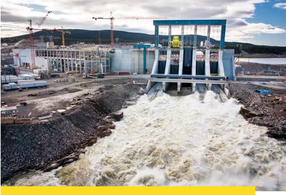
Muskrat Falls Power Generating Station, NL Canada
