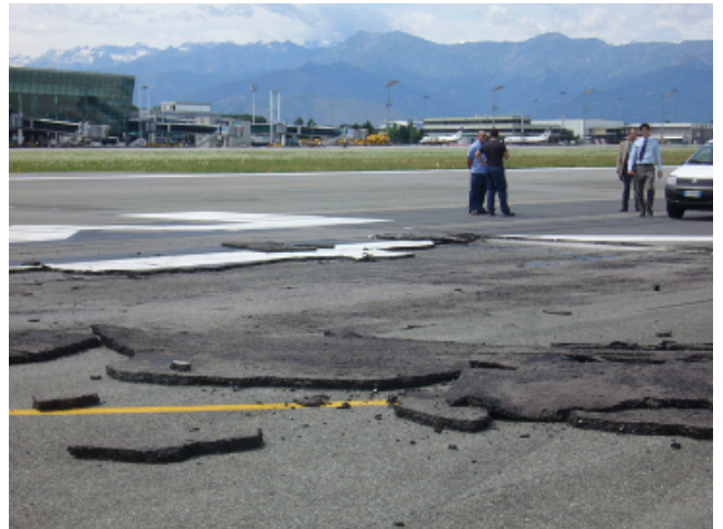
Delamination in Airfield Pavement
