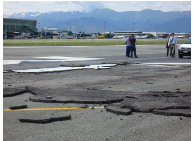
Delamination in Airfield Pavement
